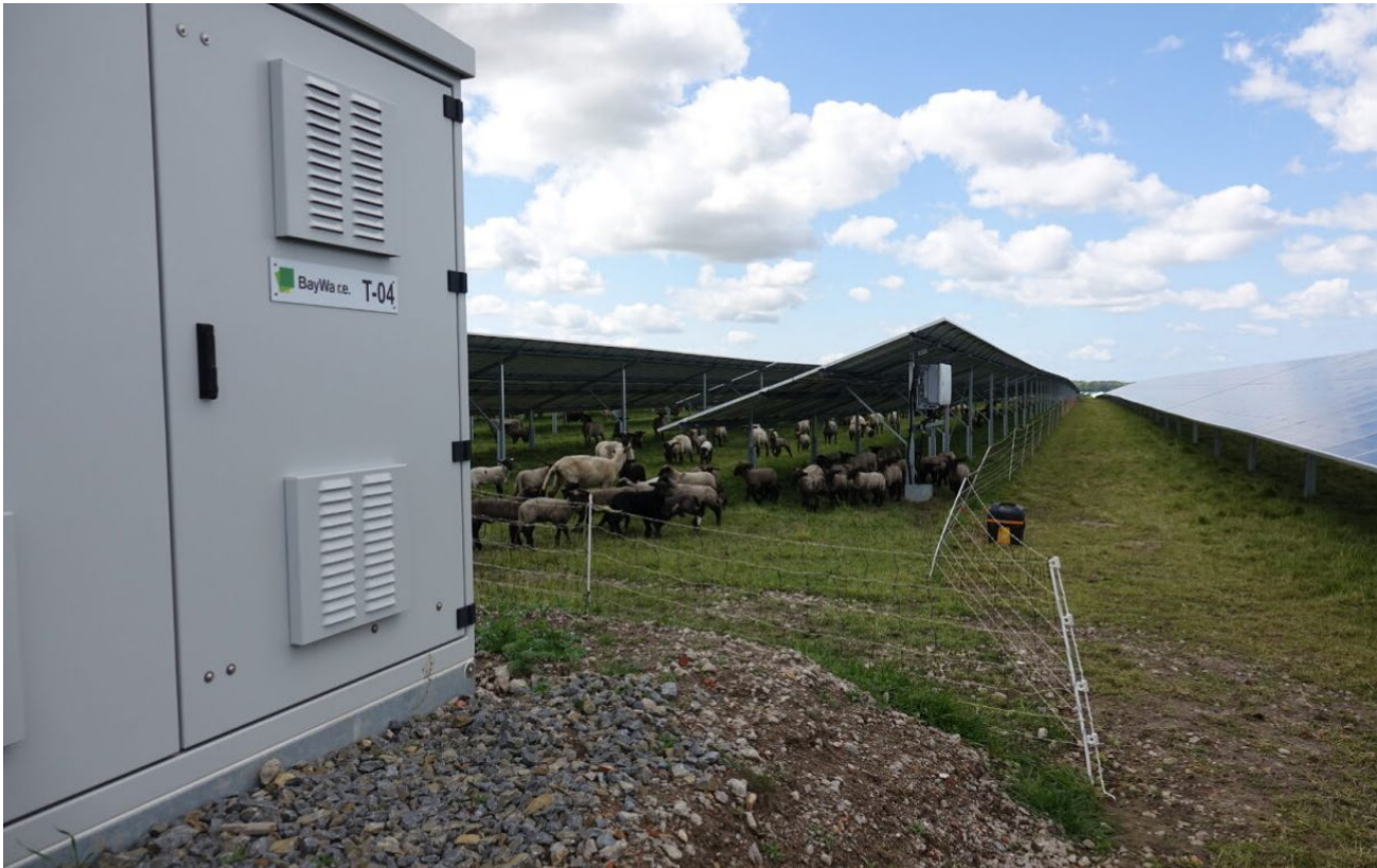
Plate 3: Typical transformer on a solar farm site
